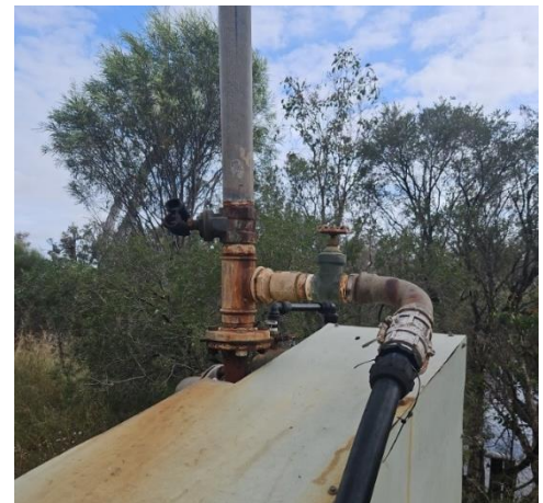
Tap on standpipe
