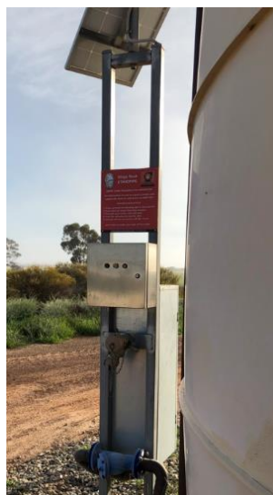
Swipe card standpipe system
