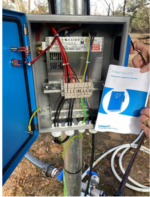
Pump panel and instruction manual. Generator can be added for flow boost.
