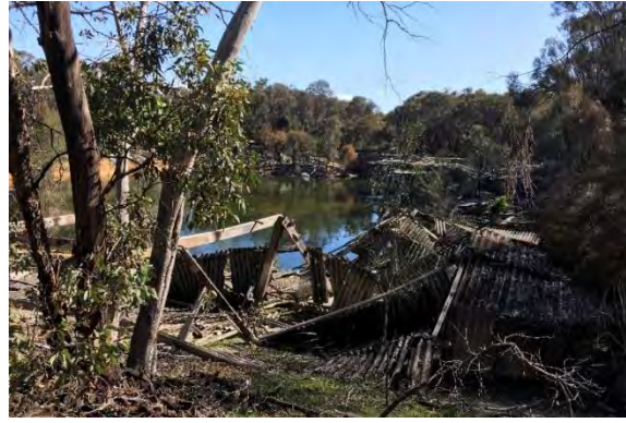
Plate 6. Hillman Dam with collapsed asbestos roofing around the edges (source: LocationsHub)
