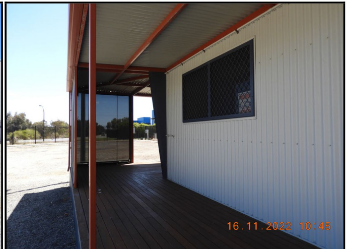
Photo 2 : Front Verandah decking is not part of the prefabricated house relocation
